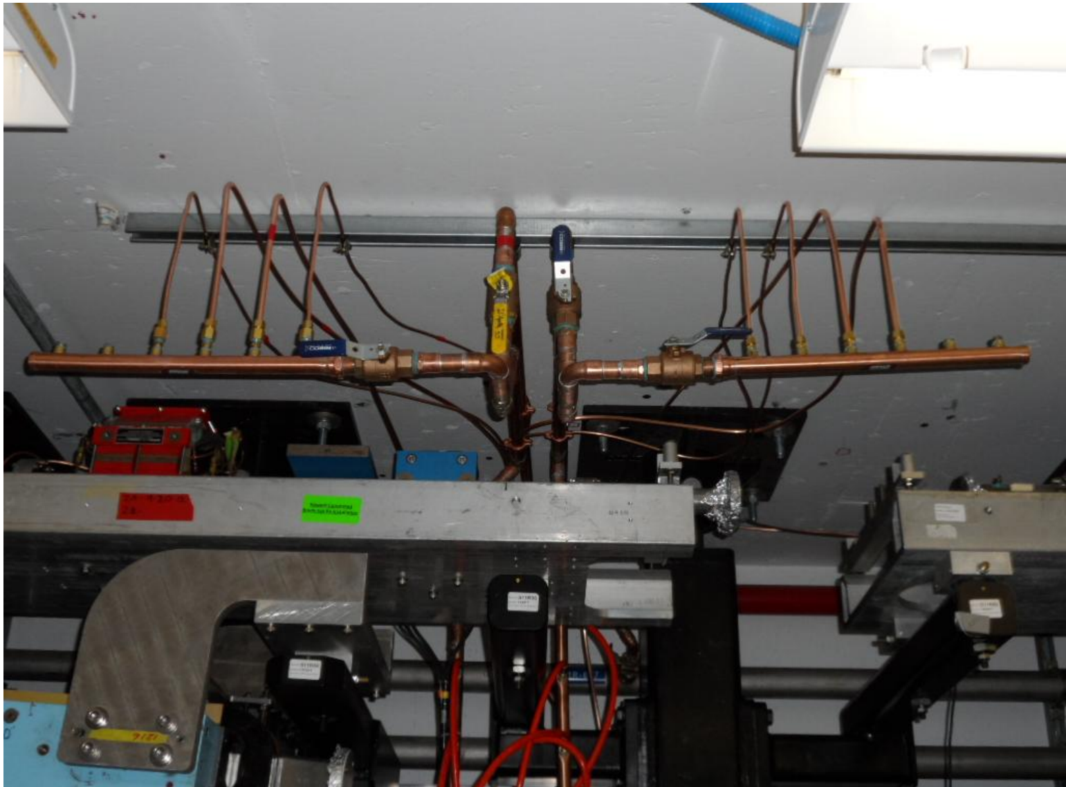
One of three 1R shunt load LCW manifolds
