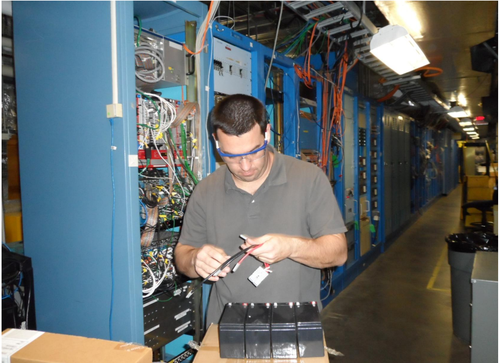
Performing PM on UPS systems
